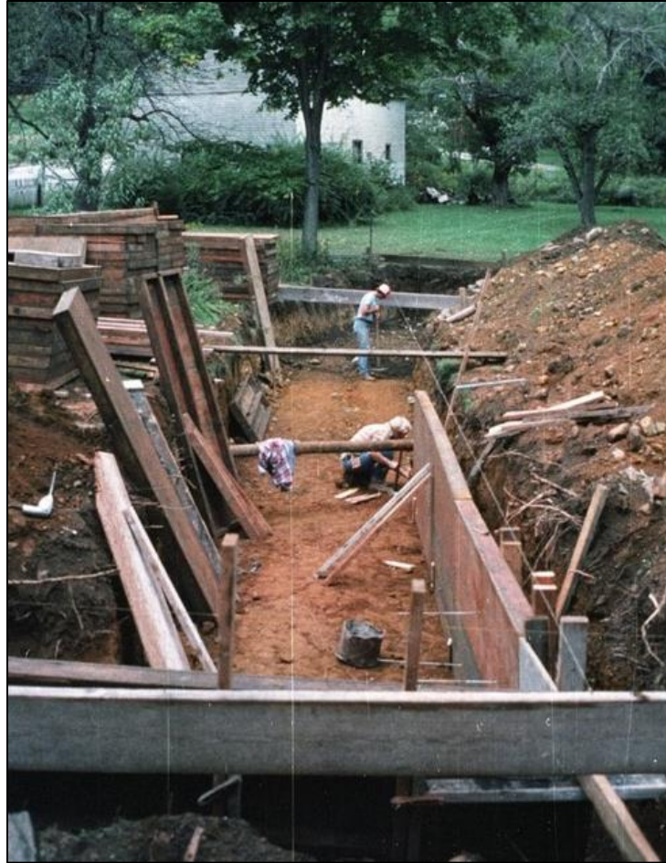
Figure 5: Photograph showing the extensive trench excavated prior to the installation of the access ramp in the early 1980s.
